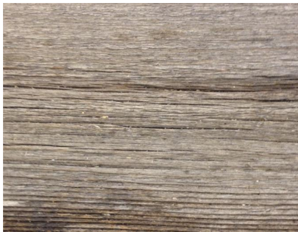
Figure 10. Surface weathered by sun and rain.
