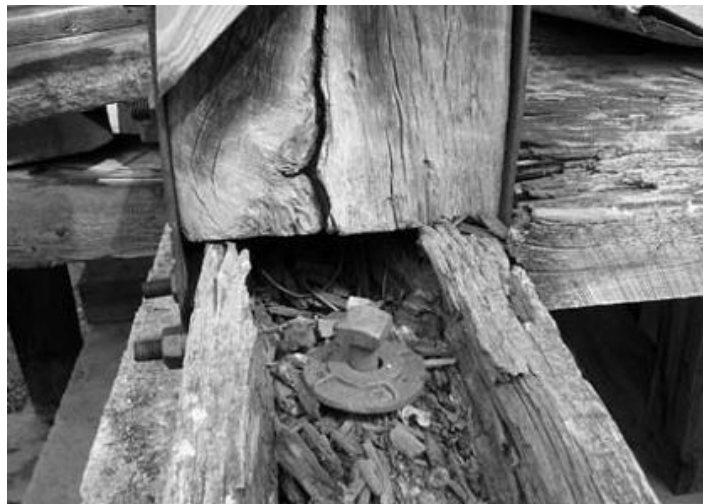
Figure 6. Decayed beam. (Anthony R. W., 2007)
