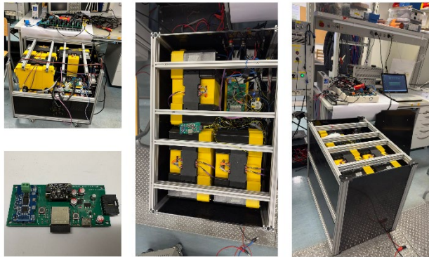
Figure 2.9 BMS configuration and connectivity, and home battery assembly and test stages in the laboratory.
