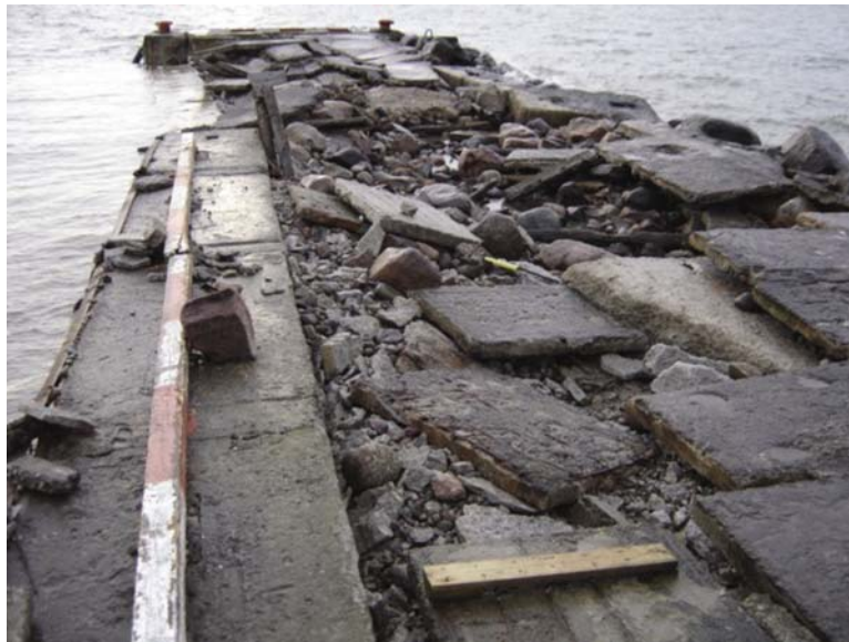
Figure 5.3 The damage caused to Aegna Harbour by the storm in January 2005 (Photo by H. Udusaar)
