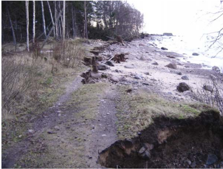
Figure 5.2 The damage to the Aegna Island coast after the storm in January 2005 (Photo by H. Udusaar)
