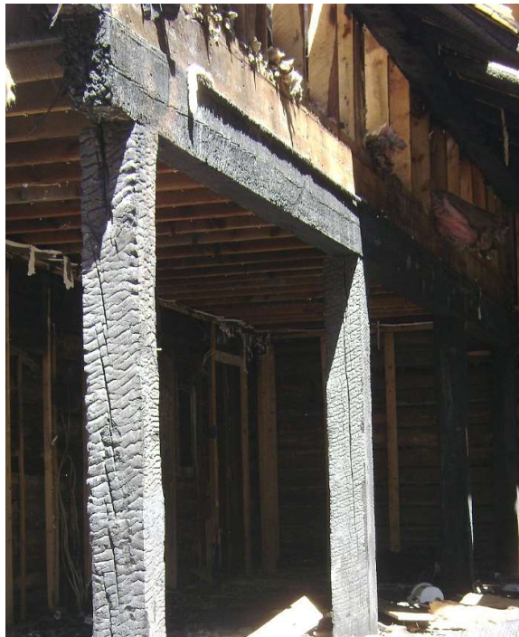
Figure 1.2 Glulam column after fire
