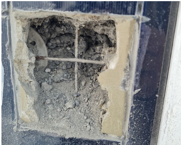
Figure 29. Destructive inspection of the reinforcement mesh embedded in the PCM mortar. Minor corrosion spots are visible to the left of the inspection opening.
