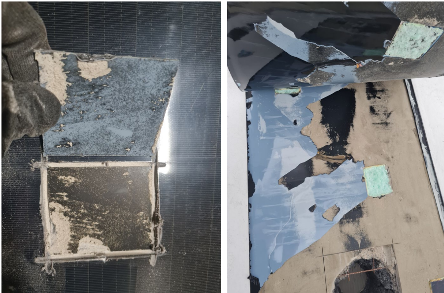
Figure 28. Delamination of the black back-side coating of the PV panel (left) and delamination occurring within the internal layers of the PV panel (right).
