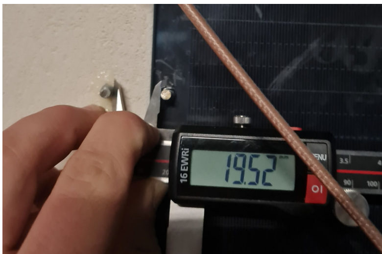
Figure 22. Measurement of relative deformations between the facade plaster and PV panel at the joint. Similar stainless steel reference tabs were used to determine the deformations of the facade plaster and the PV.
