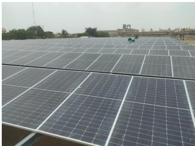
Figure 2.6 Solar units installed on roof top
