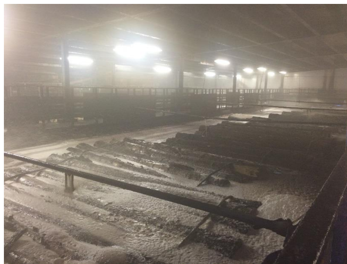
Figure 2. Water tank - (Authors photo 2015)
