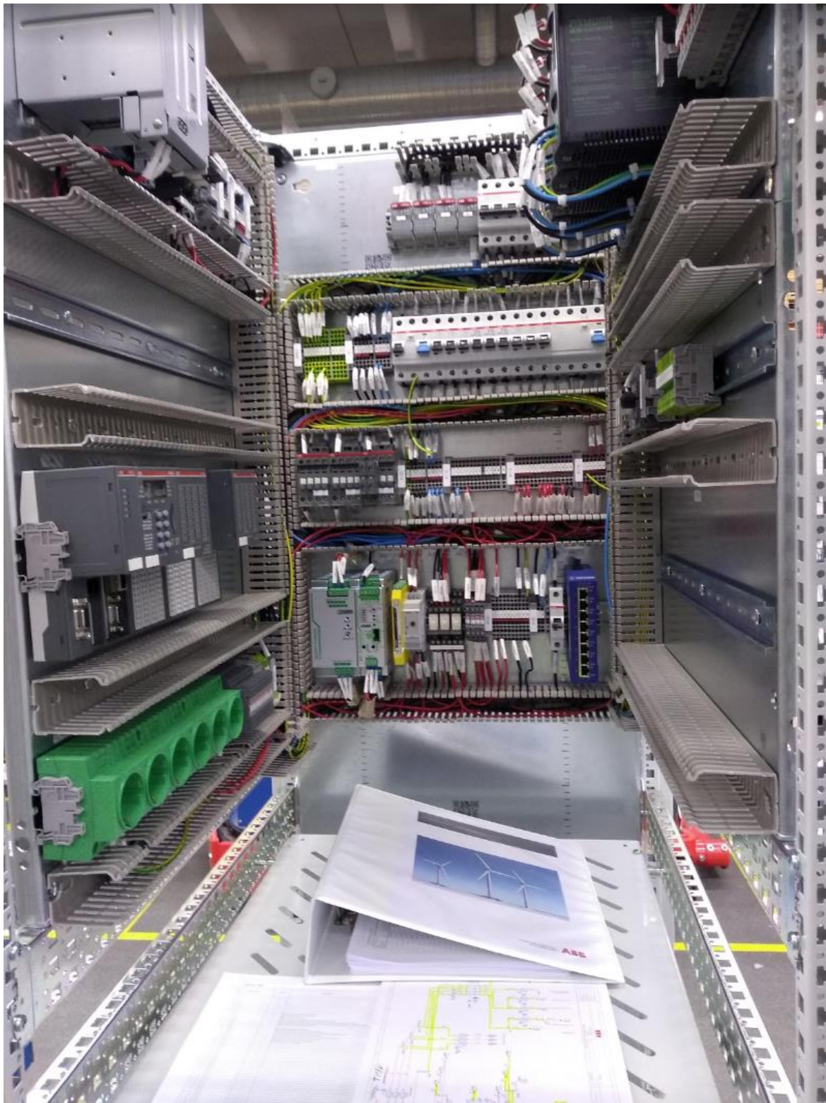
Figure 1.3 Half-finished control cabinet in production
