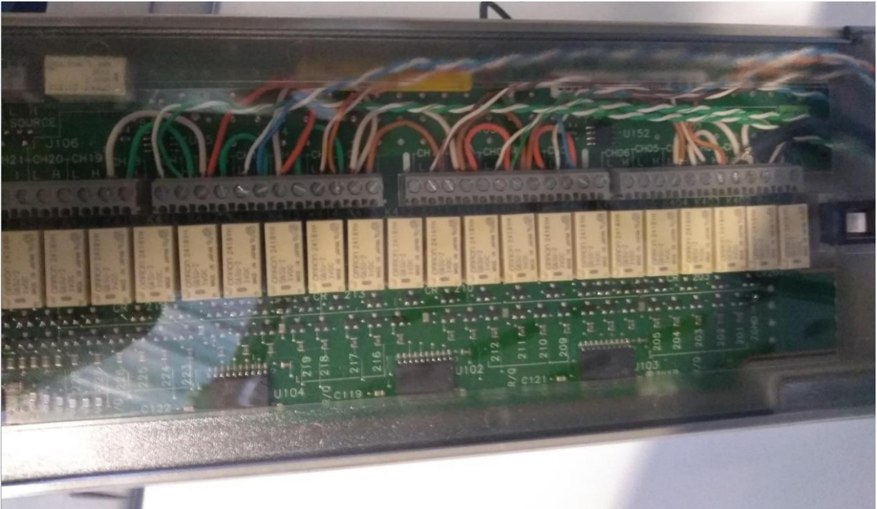
Figure 1.6 Shunt and voltage measurements connected to Keysight 34970A Data Acquisition Unit multiplexer cassette.
