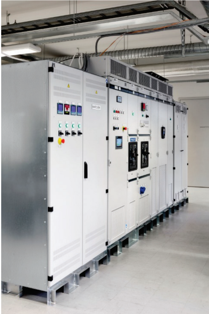
Figure 5.16 – Experimental ESS built in cooperation with the Department of Electrical Engineering of Tallinn University of Technology and Harju Elekter Elektrotehnika AS.
